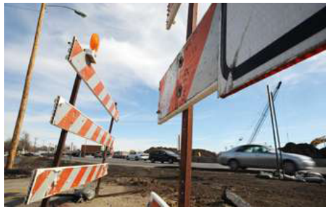
Construction continues on "O" Street as part of the Antelope Valley Project. A proposed package of new codes and design standards for the project will govern new development in a large area of Lincoln, from K and L streets north to the state fairgrounds. (Heidi Hoffman)
